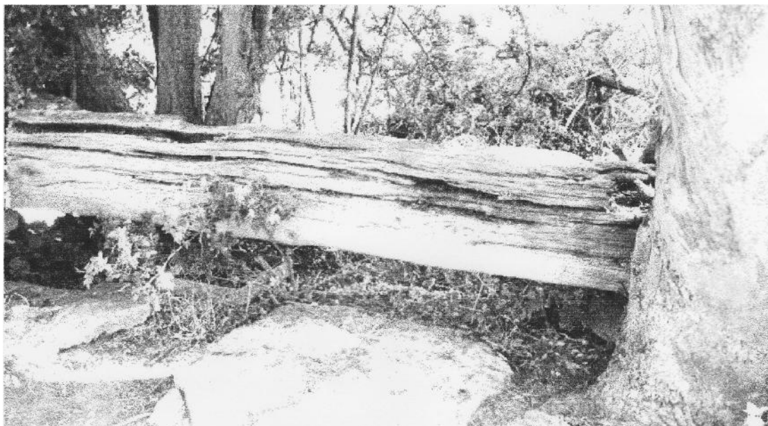
The old lock beam which has deteriorated since we last photographed it in 1997
