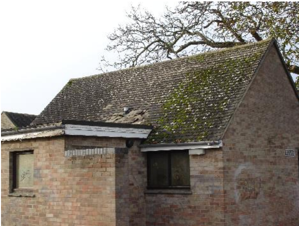
Illustration 3: Public toilets in Back Lane Car Park. Negotiations between district and parish council are still unresolved
