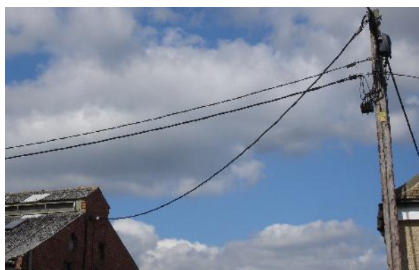
Illustration 10: Typical view of Eynsham's overhead cabling
